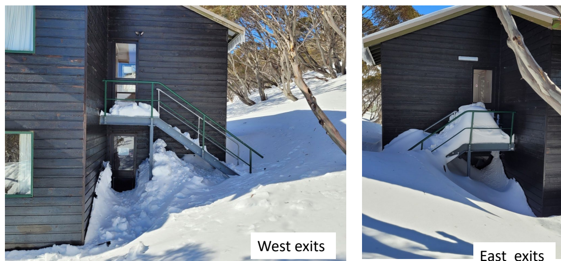
Figure 12: Rear exits on June 14 2022 showing snow build-up, particularly on east of lodge.
